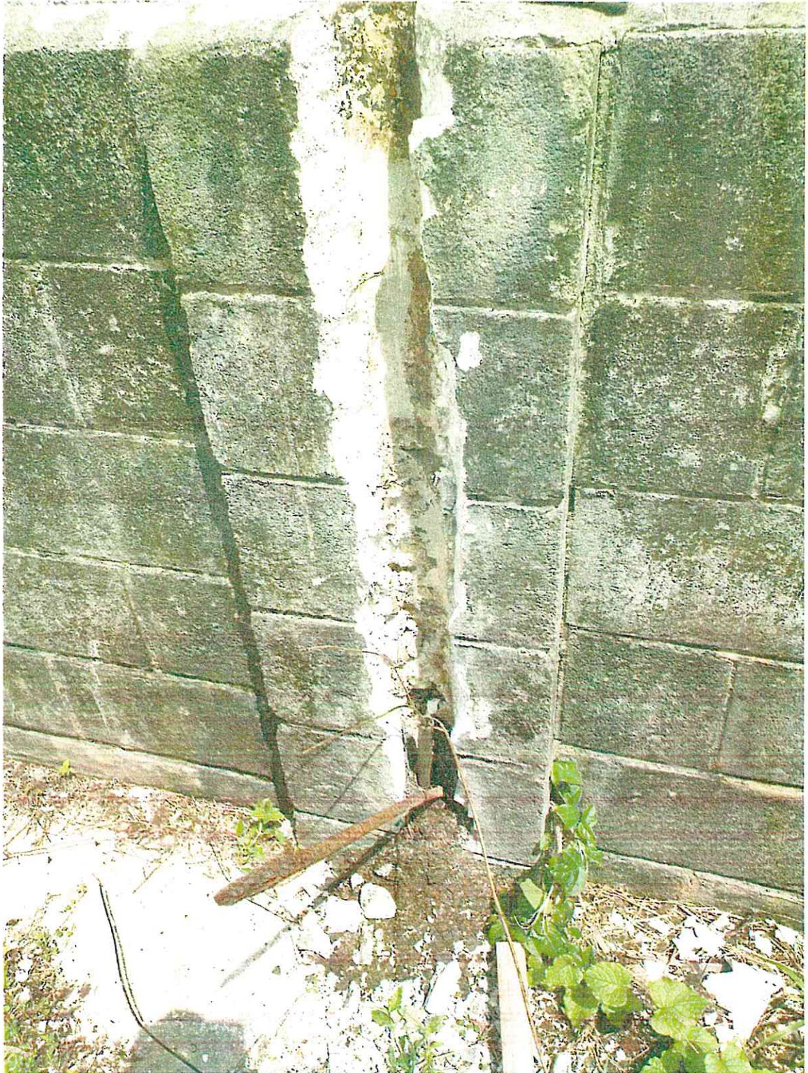
Exhibit A: Impassable conduit at Northwest parking light. Old deteriorated wires could not be removed. Rust debris from old light post visible.
