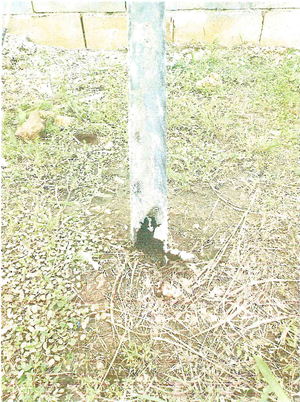
Exhibit A: Condition of light post removed from Southeast parking light. Light gauge steel has rusted entirely causing failure at pedestal.
