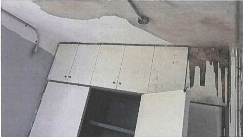
Typical existing closet partitions, shelves, doors, hardware & wood jambs damaged, mold & mildew
