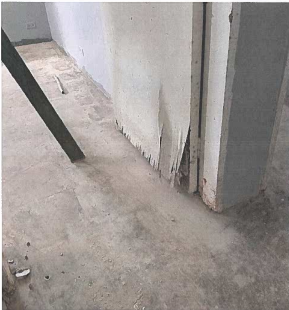
Typical interior door damaged
