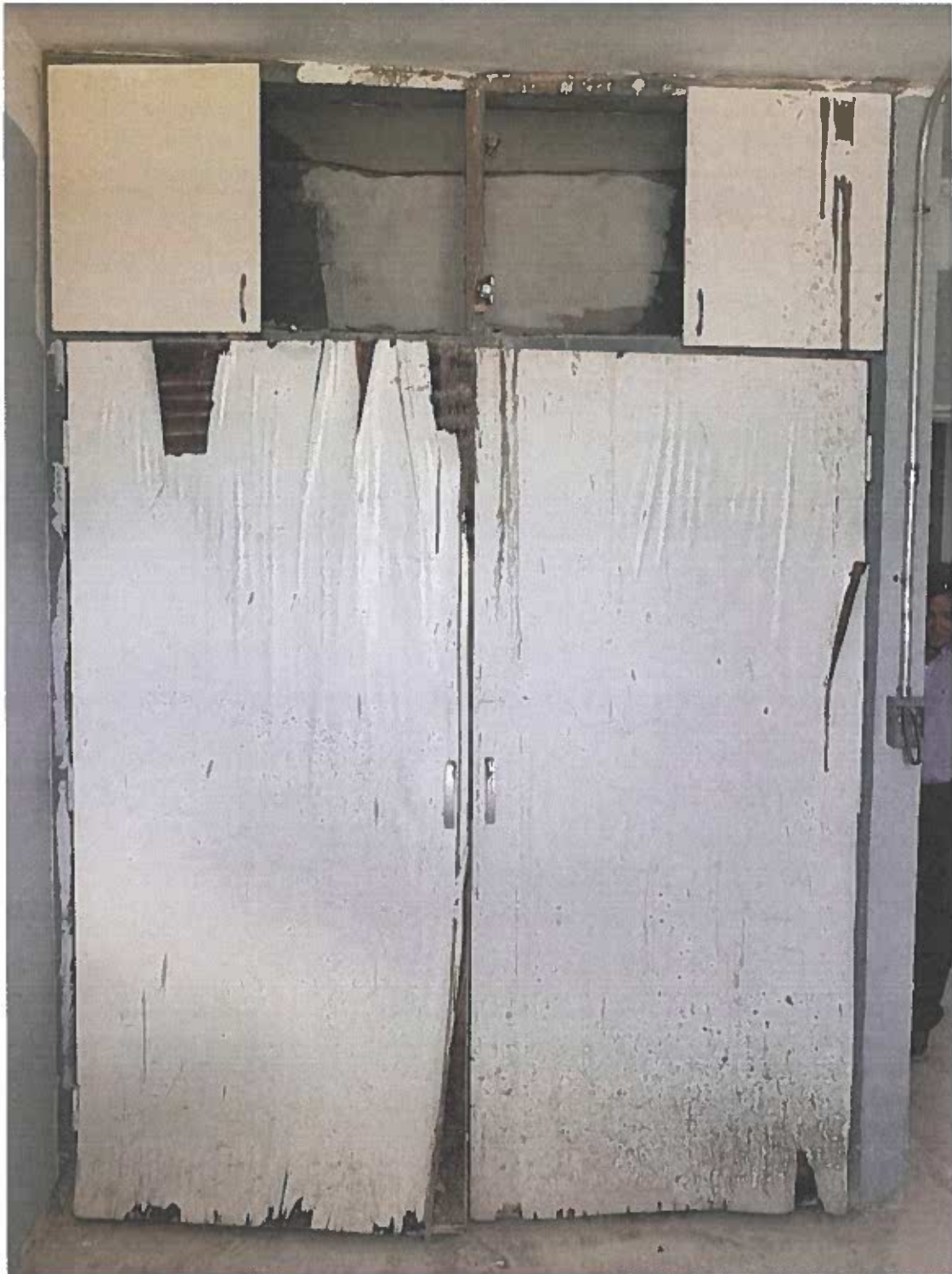
Typical existing closet partitions, shelves, doors, hardware & wood jambs damaged, mold & mildew
